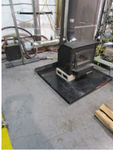
Side of heater
